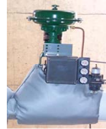
Control Valve Thermal Cover
